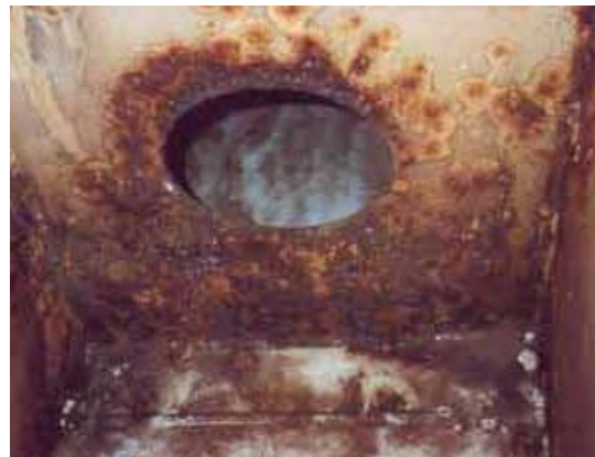
Figure 2. Actual corrosion on ballast tank.
